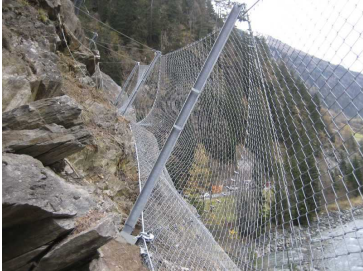
Rockfall barriers (photo Geobruigg)
