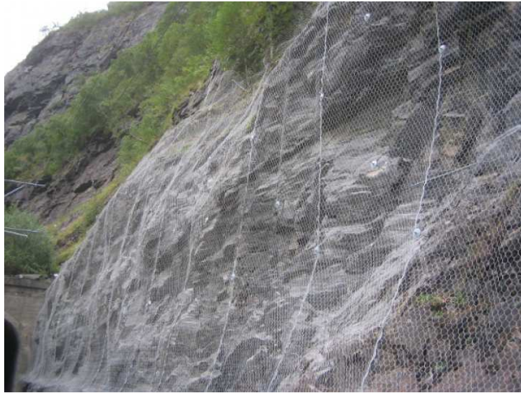
Rockfall protection nets
